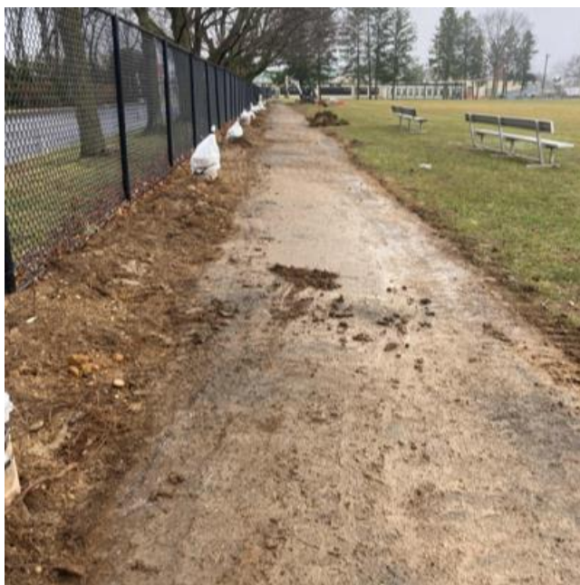
East Field House – Complete septic system and backfill, install new RPZ, install underground electric for bollard lighting
