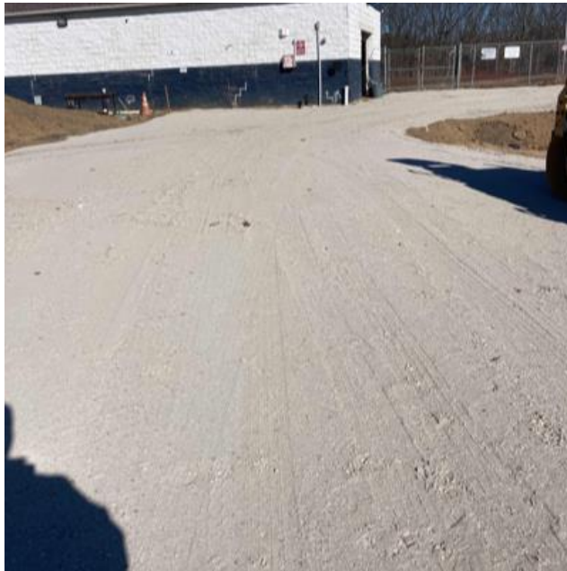
West Field House – Start and complete drywall ceilings, complete siding, prep subbase for asphalt,
